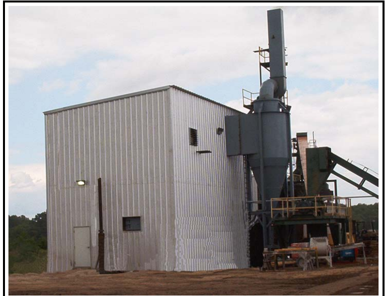
Wood Fired boiler during construction at East Mississippi Pole Company in Macon, Mississippi.
